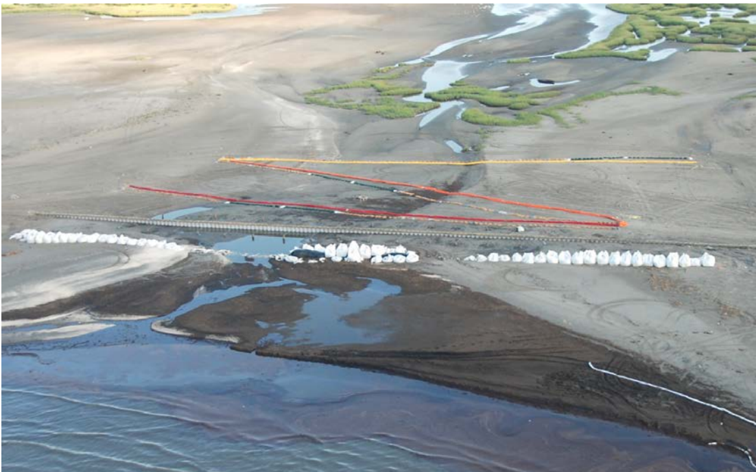
Figure 4.6 View of channel that was first protected using Super Sacks and water-ballasted booms, then with bulkhead construction. Super sacks were used at several sites as a temporary measure in advance of more permanent solutions such as bulkheads and revetments. The dark material on the ocean side water is a mixture of woody detritus and oil.
