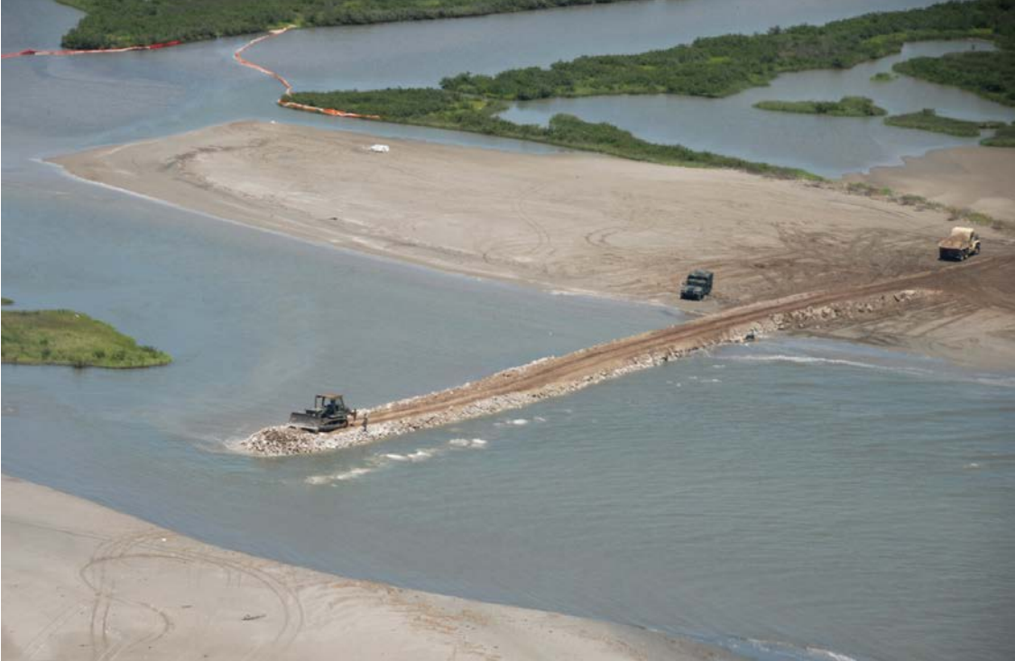
Figure 4.7A Rubble and gravel dam under construction in a 1-m deep and 160-m wide channel on a low barrier.
